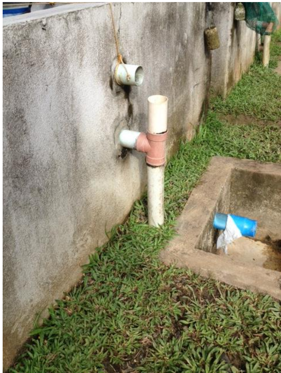
Airlift pump at outlet of tank
