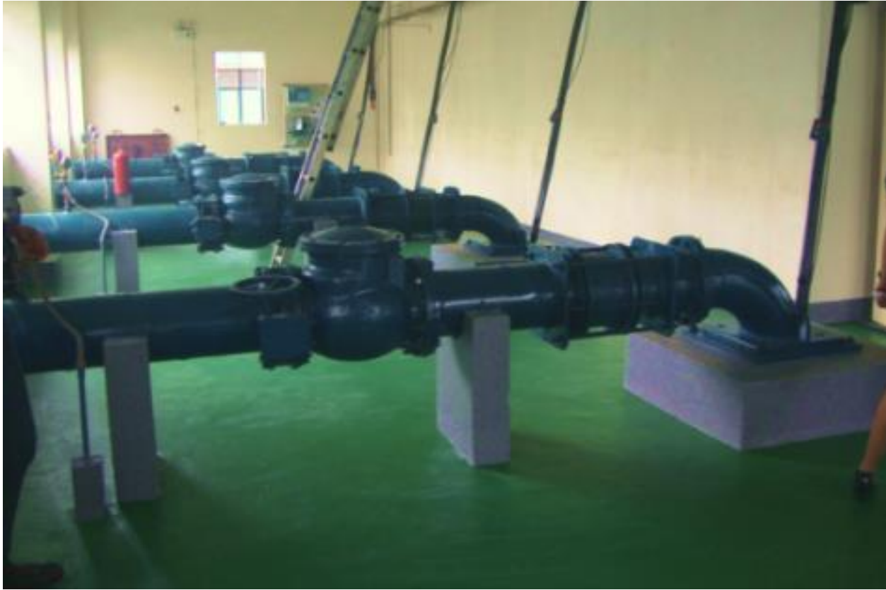
5 SUBMERSIBLE BOOSTER PUMPS during VINTA
