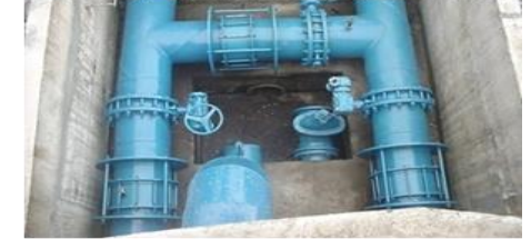
Break Pressure Tank
