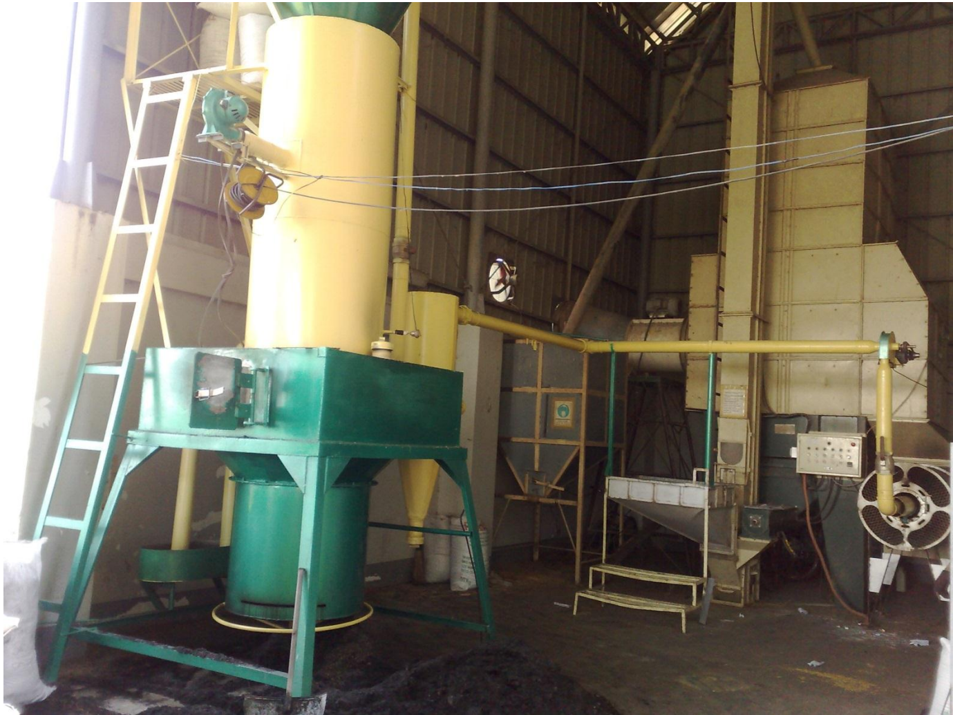
Rice hull gasifier as heat source for batch recirculating grain dryer
