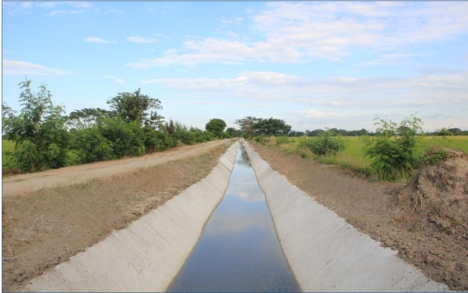
Lateral Canal with Service Road in the Mt. Pinatubo-affected SMORIS Service Area
