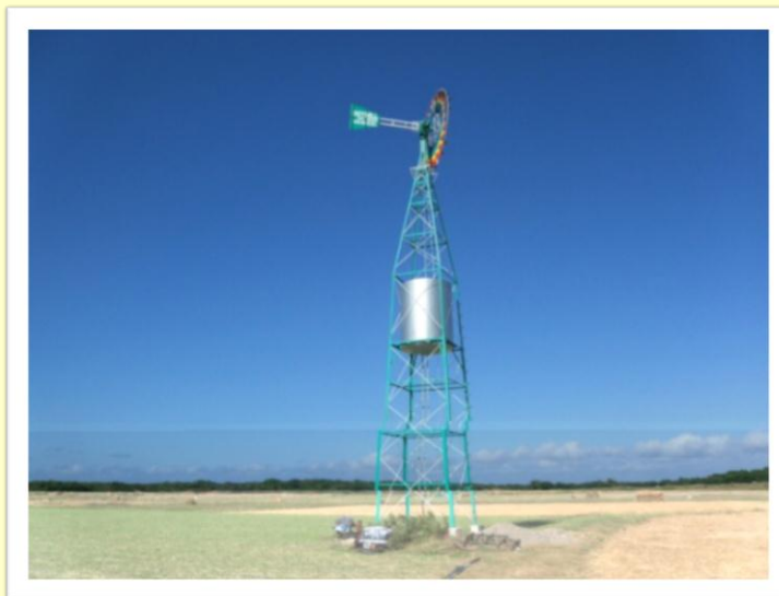
Installed Wind Pump Brgy. Bobon, Burgos, Ilocos Norte
