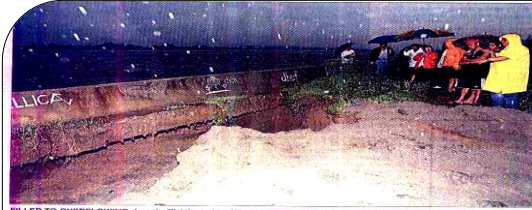
FILLED TO OVERFLOWING: Local officials and residents of Tarlac City inspect the damaged dike along the Tarlac River yesterday. The dike is being reinforced with sandbags. Floods breaching dikes; death toll hits 30 The death toll from four days of heavy rains and flooding in Tarlac City, Pangasinan, reached 30 on Monday, with four other people reported missing and 41 more injured. More than 35,000 people remained in evacuation centers, although floodwaters in some areas were subsiding. Abandoning rains were expected to continue over Southern Luzon. Initial damage estimates from the flooding and torrent rains have reached P14 million, according to the office of Civil Defense. In Baguio, the subposed industry lost P75 million. While public and private institutions maintained full operations in Baguio, according to the provincial division of management & contracting office. Alberto Reyes, a former official of the Bureau of Fire, said in Manila, and the main source of flooding in the capital town of Tarlac and the surrounding area. The establishment of business establishments of private business prior to rain. In Tarlac, Gov. Jose Nepomuceno ordered sandbags placed on the banks of the Tarlac River to protect the city's main market and south-western Tarlac city from overflowing floodwaters. The Tarlac River has been serving as a sink basin for floodwaters from the mountain range of Central Luzon. Reports said cascading floodwaters from Mt. Pinatubo and the western mountain ranges of central Luzon have washed across the dike, that have been keeping the Tarlac River from overflowing and flooding nearby barangays. Who have been flooded with respect to evacuation centers for sandbagging operations. Virgilio Berrera, office in charge of the Tarlac provincial disaster coordination center. Floodwaters have submerged nearly all of Barangay San Mateo and about half of neighboring barangays south of Tarlac City, with flooding about 100 meters. Turn to p.
